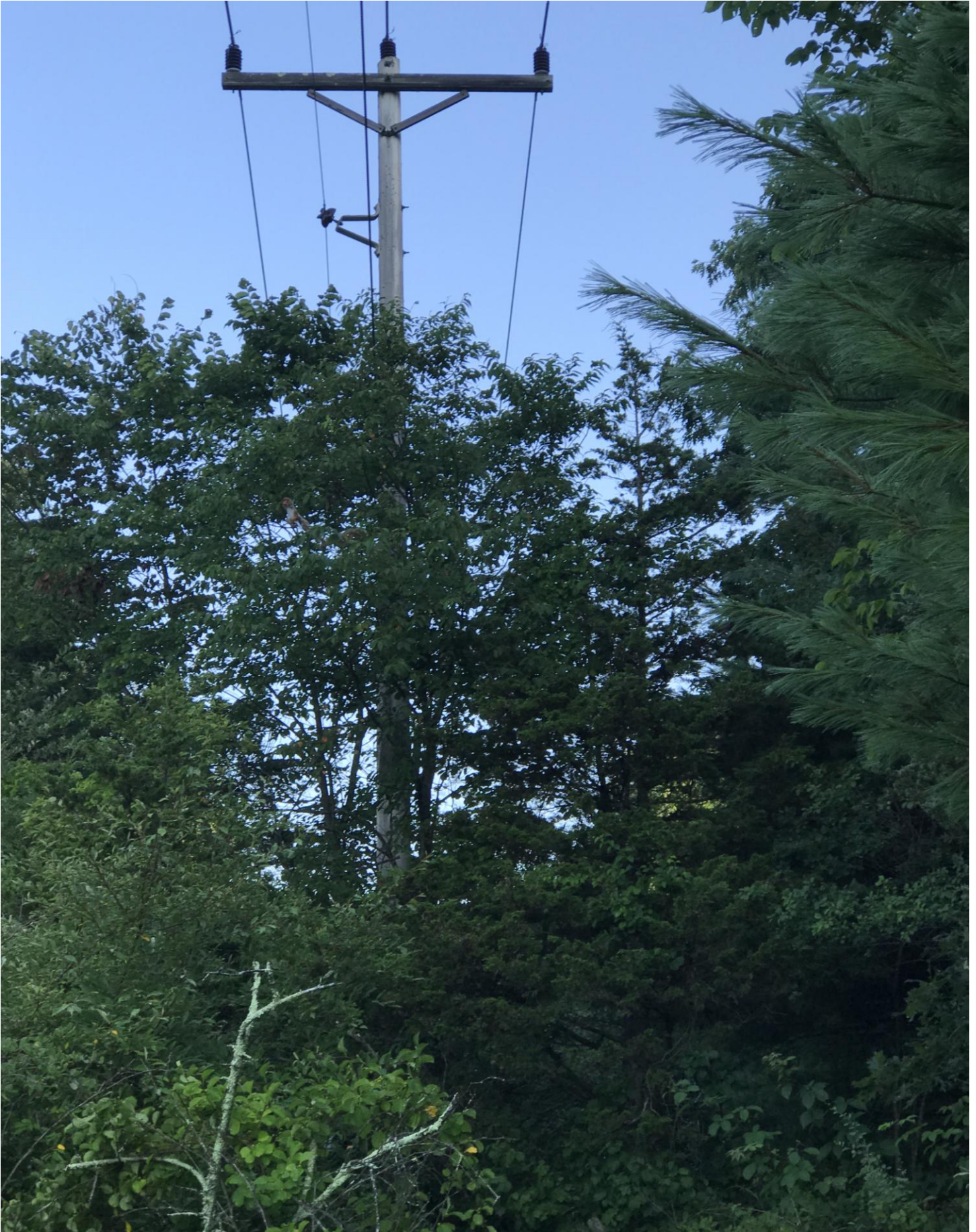
Current vegetation growth around lines, equipment, pole on Fitch property August 15, 2019 - B
